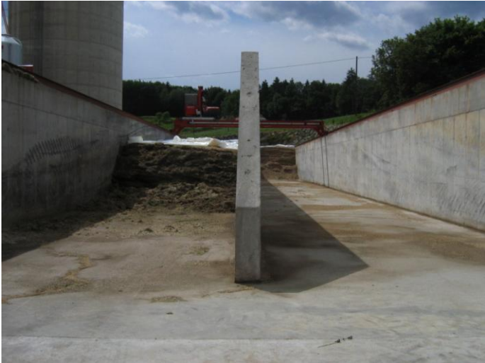
Photograph 6.5: Two drive-in open silos for maize and grass silage
