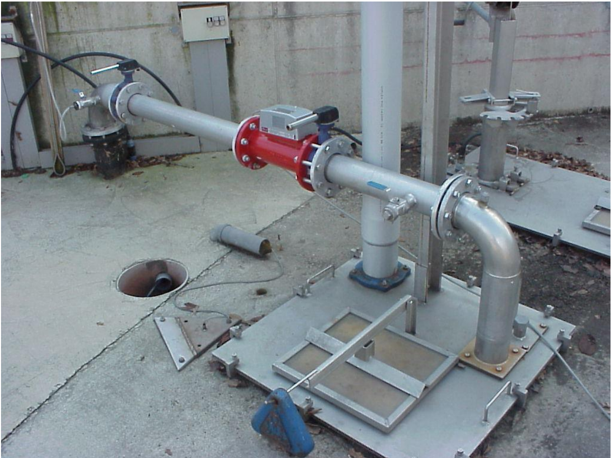
Photograph 6.8: Biogas flow meter of company ESTERS Elektronik, Type 005 GD 100 / with data processor GVPA-303-GDR, for measurements of the biogas flow from the storage to the other part (secondary digester) of the biogas plant.
