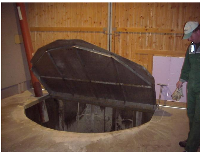
Photograph 6.3: Underground mixing tank of Biogas plant Paldau
